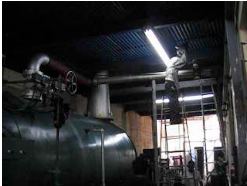
400 hp Cleaver Brooks Boiler in El Salvador
